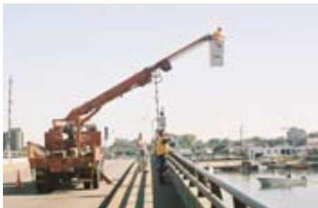
Consultant and WisDOT engineers use a bucket truck to determine optimal positioning for the elevated cameras on the Wisconsin St. Bridge in Oshkosh.
