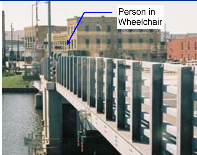
Photo from bridge tender house showing person in wheelchair near bridge railing. Note how person in wheelchair is obscured by railing.
