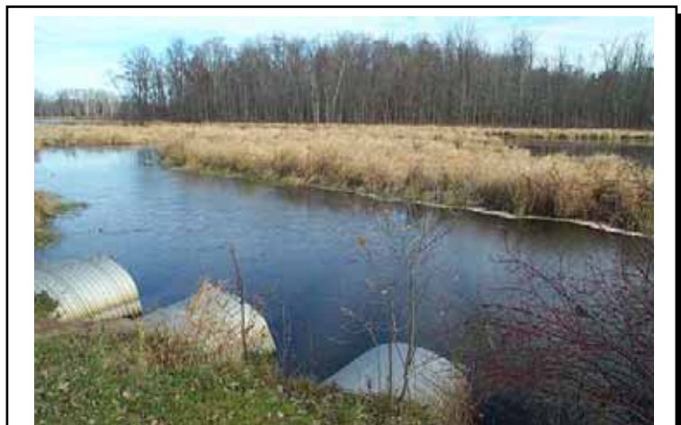
Figure 3.1-6 East View of Black Otter Creek South of WIS 15 at Equalizer Pipes. Floodplain Area is Reportedly Groundwater Discharge Area
